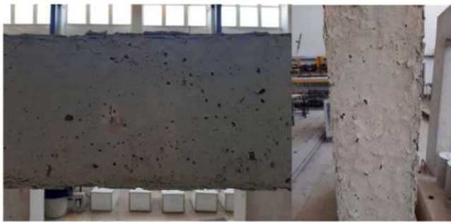
Fig. 7. Blistering and spalling on the concrete surface.
